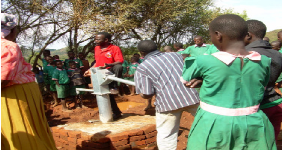
Students at Malanga Primary school listening to the driller's explanation when fixing the water pump.
